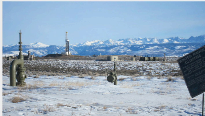
These pipelines are part of the heavy industrial natural gas field in the Pinedale Anticline. (Dustin Bleizeffer/WyoFile – click to view)
